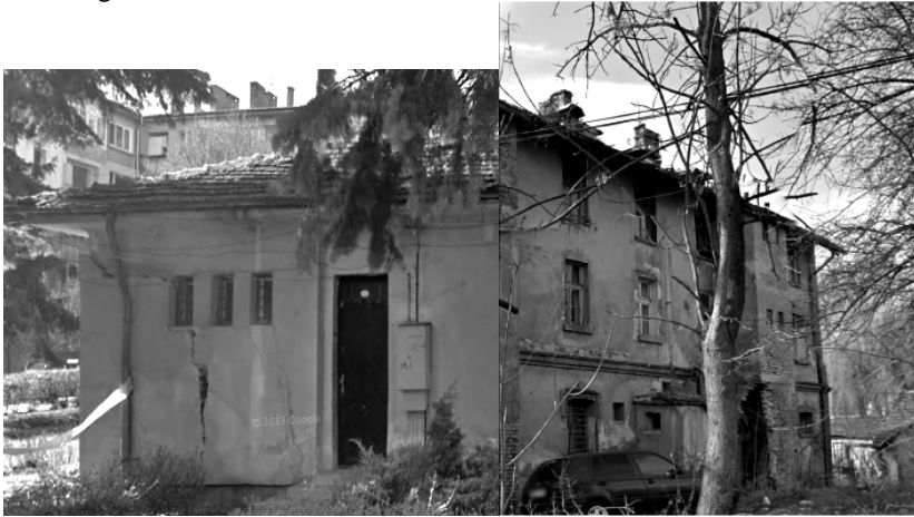
Fig.2. Buildings with damages from 7-8 degree
